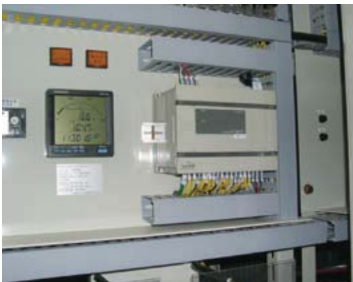
Energy measurement system
